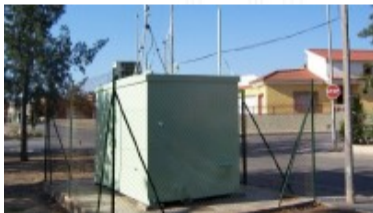
La Aljorra monitoring station. Source: Google Images
